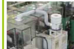
Oil mist collector mounted on a machine tool
