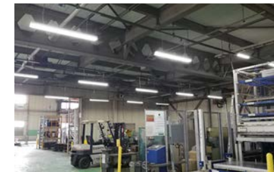
New LED lamps (Hosoe Factory)
