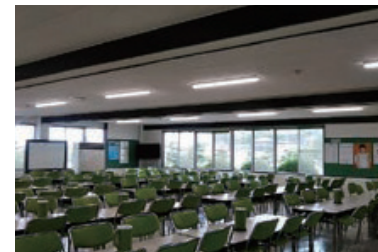
New LED lamps (Hosoe Factory)
