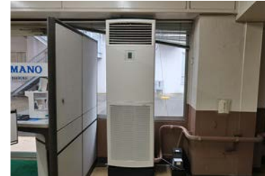
Renewed air conditioners (Head office)
