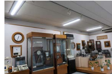
New LED lamps (Head office)
