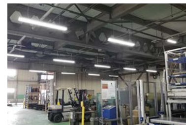
New LED lamps (Hosoe Factory)
