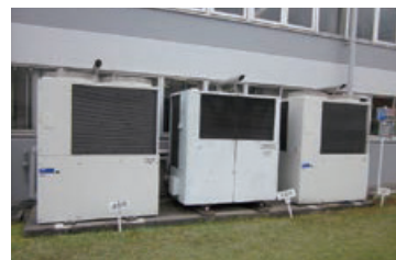
New GHP air conditioners (Hosoe Factory)
