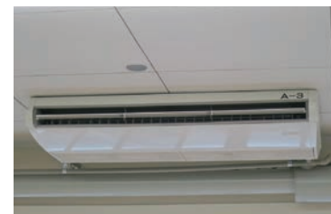
Renewed air conditioners (Head office)
