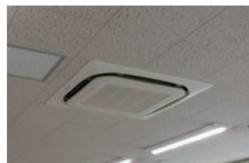
New air conditioners (Sagamihiro Factory)
